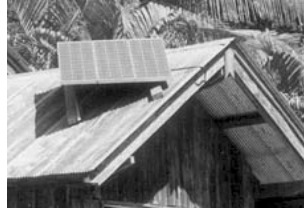
Figure 6: Solar Panels Mounted on a Roof
